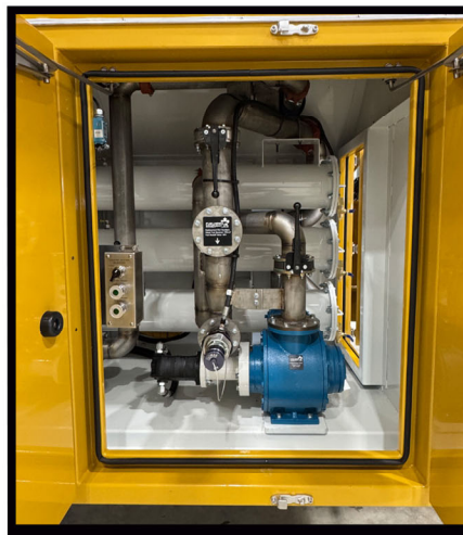
RH Side Diesel Fill Cabinet
