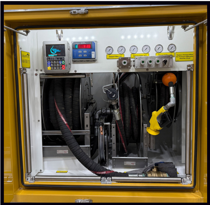
Diesel Dispense Cabinet
