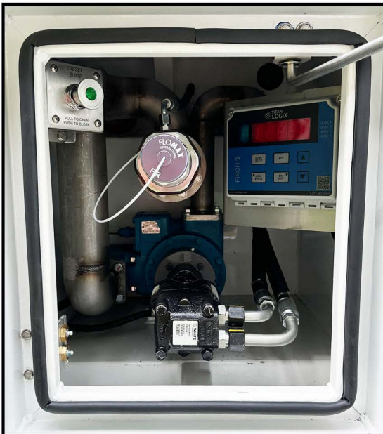
Passenger Side Fill Port Cabinet
