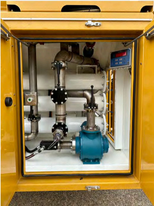
Diesel Fill Port Cabinet
