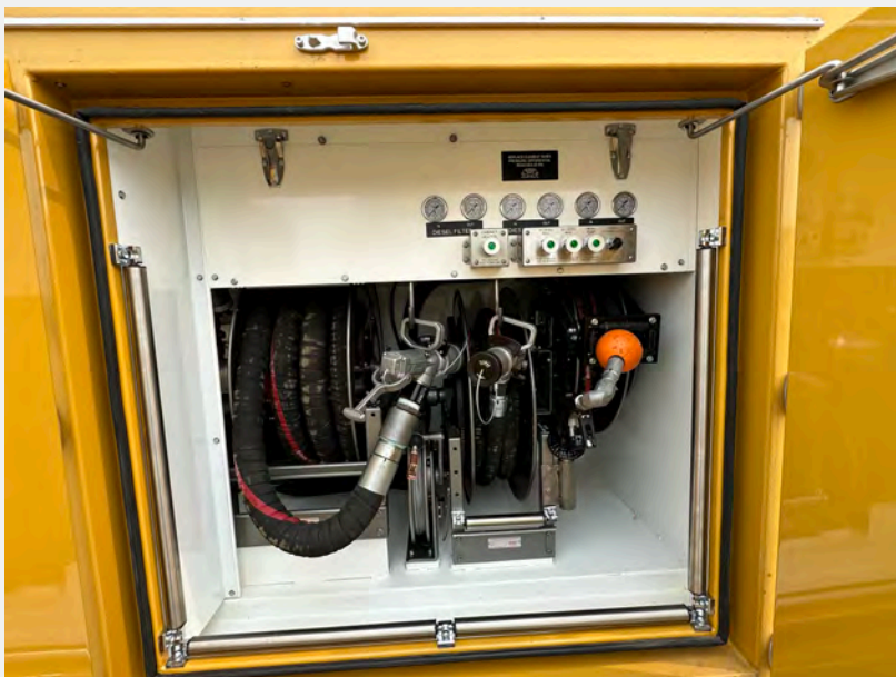
Diesel Dispense Cabinet
