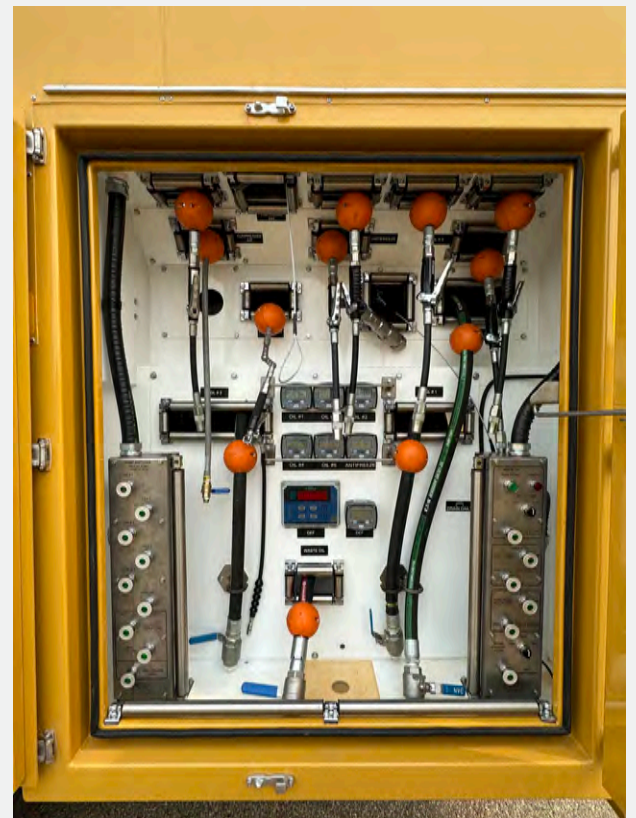
Lube and DEF Dispense Cabinet
